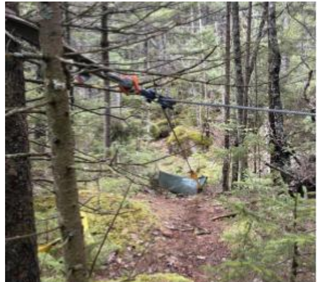
A retired canoe and Griphoist rigging system transporting bridge stringers to Katahdin Stream Falls
