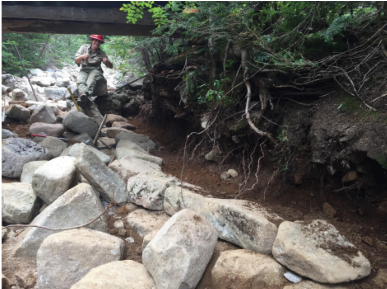
Figure 3. The first tiers begin to take shape underneath the Upper Saddle Brook Bridge
