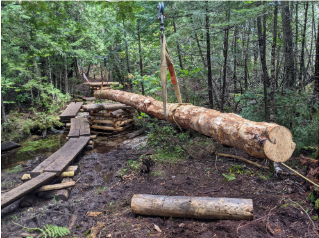
Figure 5. Spruce bridge stringer is high-lined into position to form the ramp of the new OJI bridge crossing.
