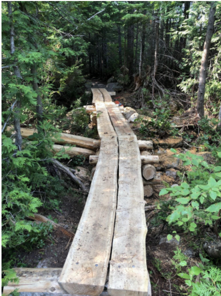
Figure 4. A newly rebuilt section of elevated bog bridging on the Chimney Pond Trail
